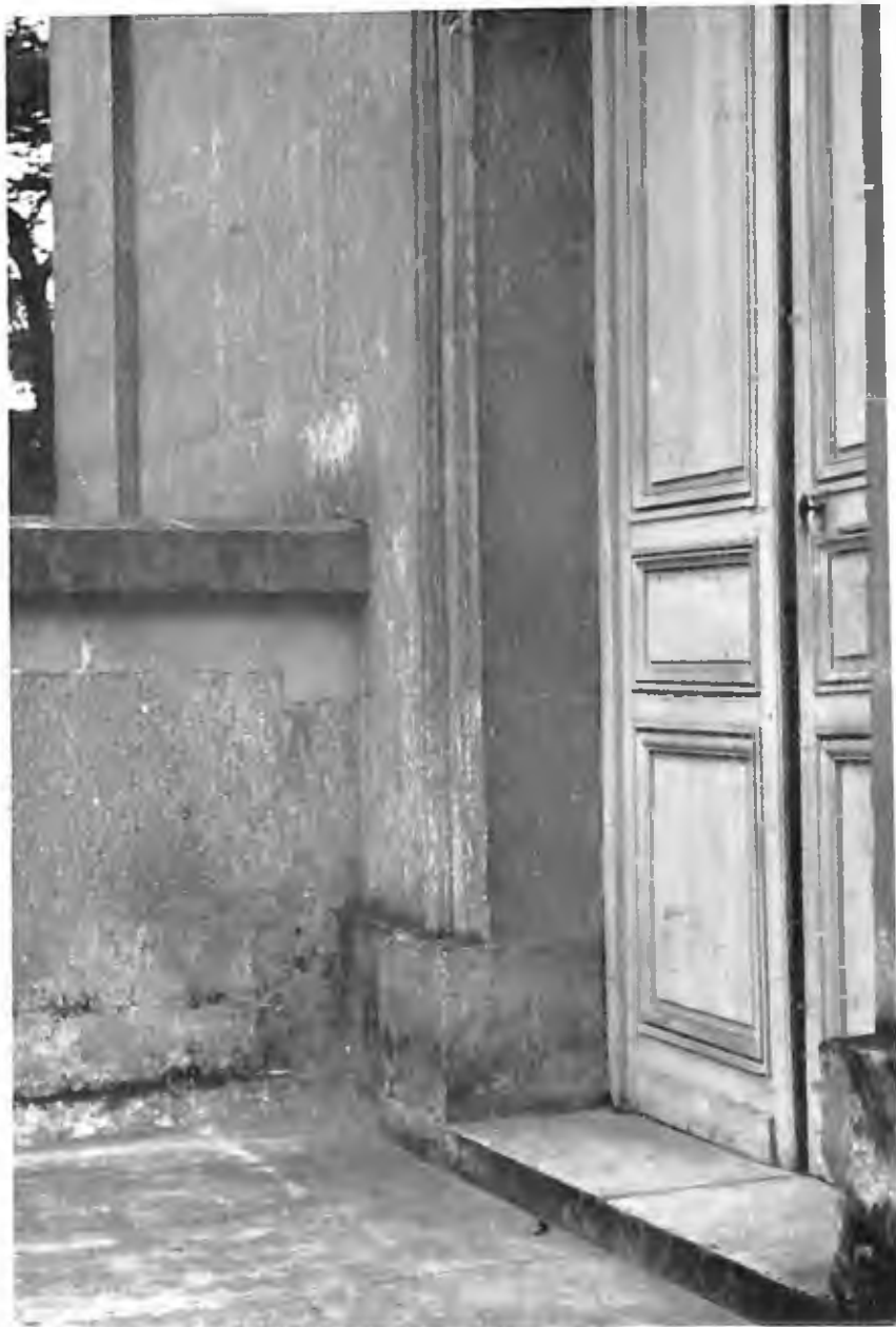
18. Detail of the Chapel Doors and Terrace Pre-coved stone flags turning the corner of the Chapel perron , upon which the walls are set. Mique may have cut through here to commence a communicating way to the maison (see Plate 19).
